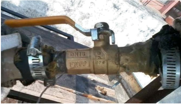
Fig. 7 Photograph of the gate valve
